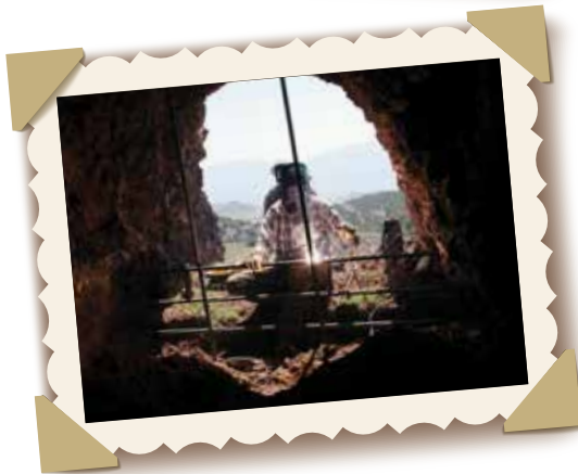
Check out our Abandoned Mine Reclamation team hard at work preparing a site and building a bat grate.
