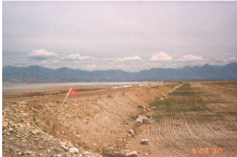
Figure 1.16: A dike is used to isolate the tailings cell. Seed is placed into amended tailings. Kennecott Tailings Facilities.
