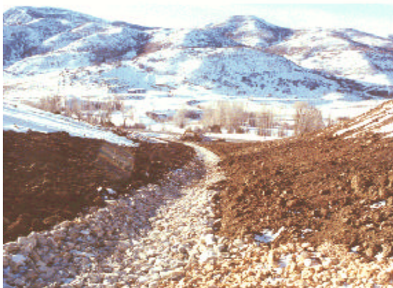
Figure 2.10: Riprap is rock with a specific mixture of sizes or gradation, used to stabilize drainages. Boyer Mine.
