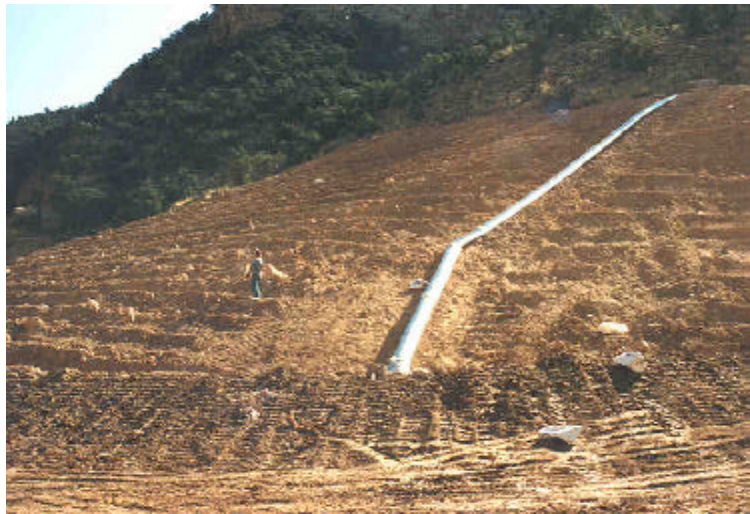
Figure 10.2: Slope drain used to convey drainage over newly reclaimed slope. Horse Canyon Mine.
