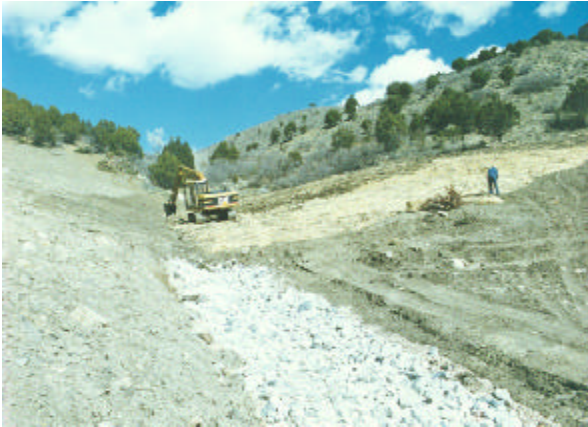
Figure 2.12: Construction of a buried channel begins with a well-constructed riprapped channel. Boyer Mine.
