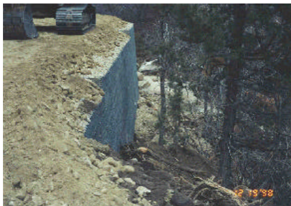
Figure 1.2: A hilfiker wall is used to construct a substation, reducing land disturbance. Dougout Mine.
