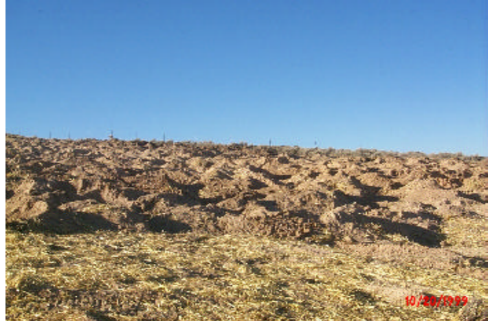
Figure 1.1: Straw is incorporated into the soil when roughening the soil surface. Crawford Mountains Phosphate Mines.
