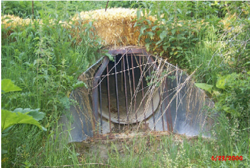
Figure 12.2: Trashrack installed to protect debris from entering the culvert. Horizon Mine.
