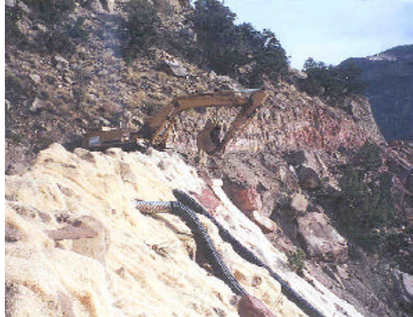
Figure 4.1: Excelsior matting is laid loosely over the seeded slopes. Bear Canyon Mine.
