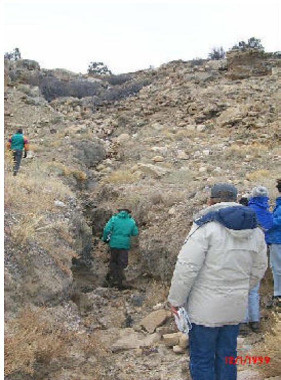
Figure 3.21: Uncontrolled erosion in unconsolidated reclaimed drainage. JB King Mine.
