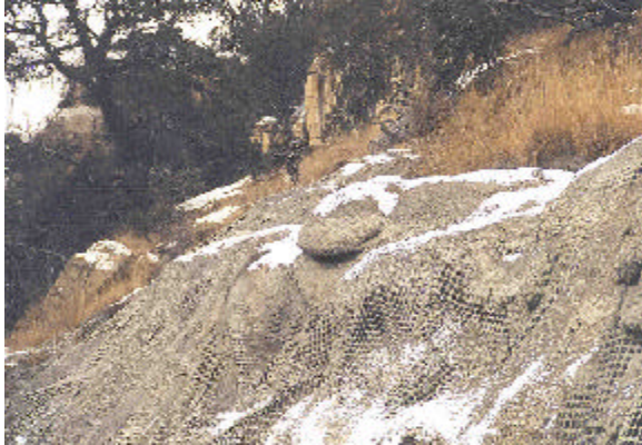
Figure 1.4: Wire mesh and gunnite stabilize the slope during the operation phase of mining. SUFCO Mine.
