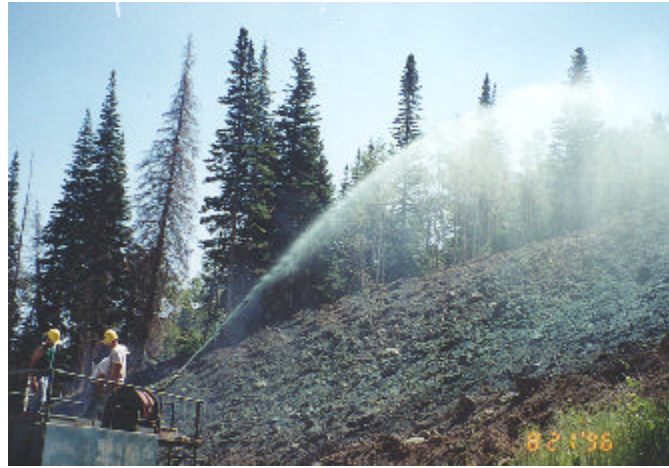
Figure 3.5: A wood fiber mulch is sprayed on the soil surface with a hydromulcher. Gordon Creek 2, 7, & 8 Mines.
