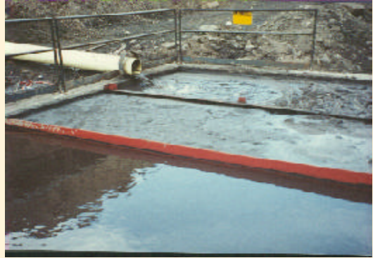
Figure 15.2 A sediment trap with baffles is used to treat water to entering the sediment pond. Deer Creek Mine.
