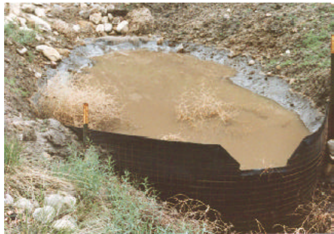
Figure 14.1: A temporary sediment basin located in a small drainageway using filter fabric. Willow Creek Mine.
