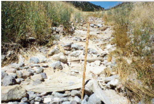
Figure 2.11: A cloth filter blanket liner is exposed after flows in this ephemeral channel. Knight Mine.
